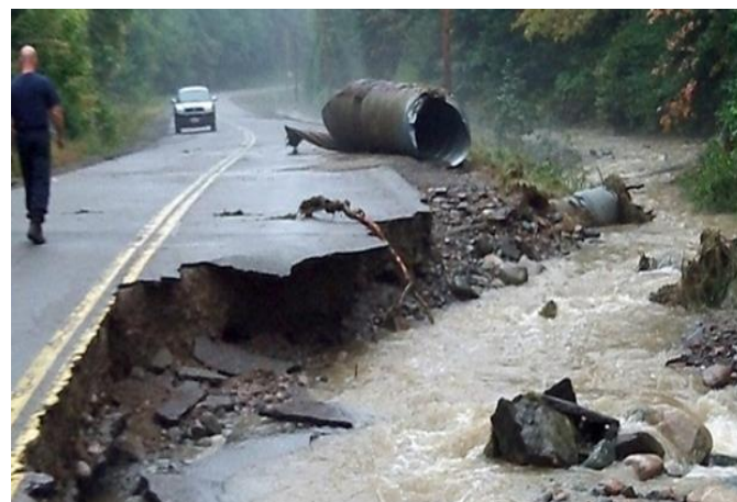
Figure 1: Damage to Highway 552 in northeastern Ontario after a heavy rain event (CBC News, 2013)
