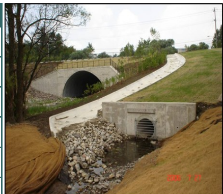
New overland flow system for Black Creek in Toronto. This was designed to prevent flood water from accumulating on the road and to prevent it from overwhelming the culvert capacity. It was built in response to the 2005 storm that washed away sections of Finch Avenue.
