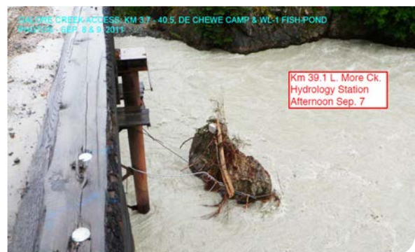
Figure 3 (top) | Flooding of access road
