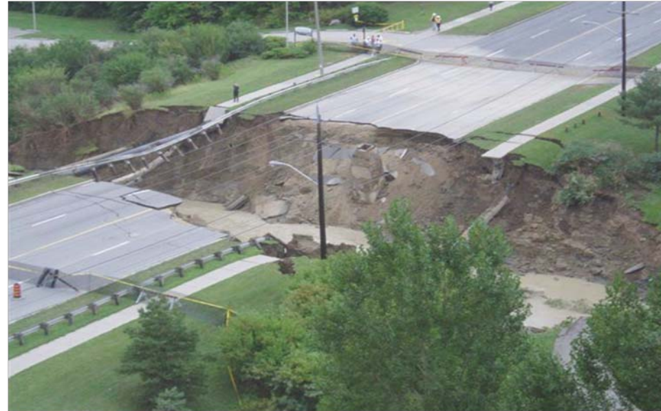
Finch Avenue Collapse, August 19, 2005
